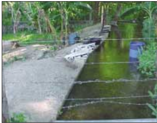
An irrigation canal which is being repaired as a result of the hydroelectric projects.
